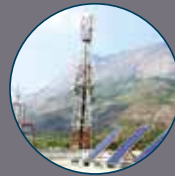
Amrita Wind Energy Centre
